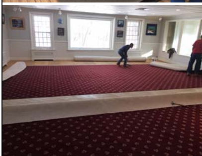
Carpeting in the Lakeside Gallery Dining Room and in the Moses meeting space getting installed by Arrow Carpet. Thanks Fred! It is beautiful!
